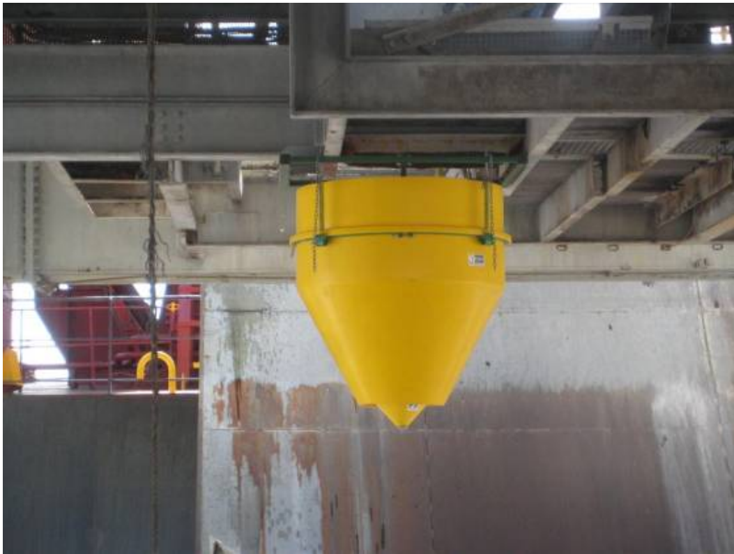
Figure 1: This is the initial height the hopper was installed prior to loading the first truck
